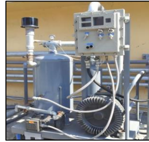
Soil Vapor Extraction
