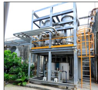
VOC Recovery System
